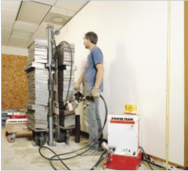
PQ603 pump and C256C cylinder used to drive piers to lift and stabilize building foundation.
