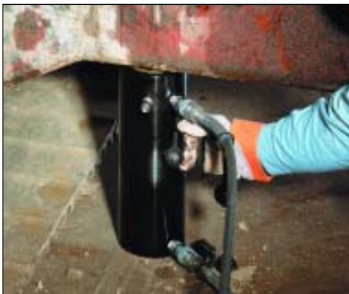
◀ An RAR-308 was easy to position under a bulldozer for repair of frame member.
